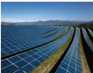
Centralized ground power station
