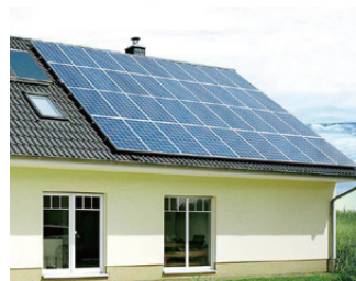
Domestic rooftop power station
